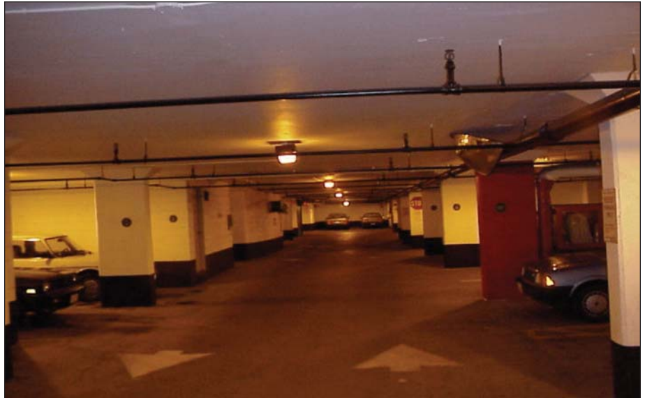
Figure 2. New garage lighting
