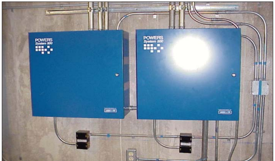
Figure 3. New building automation system
