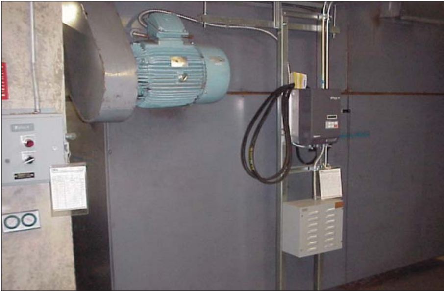
Figure 4. New fresh air supply fans
